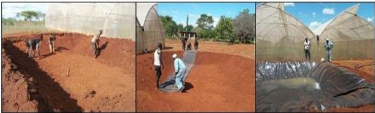
Establishing a small fishpond (left to right): 1) excavating and smoothing the pond, 2) spreading the PCV liner and burying the edges, and 3) filling the pond
